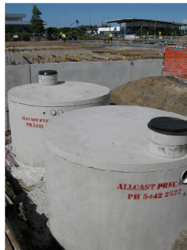
2 x 18,000Lt water storage tanks for commercial site Maroochydore
