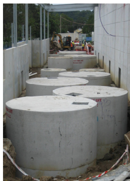
Multiple tanks for sewage system Mullumbimby NSW
