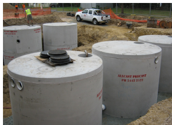
Retention/ Detention tanks—Yeppoon
